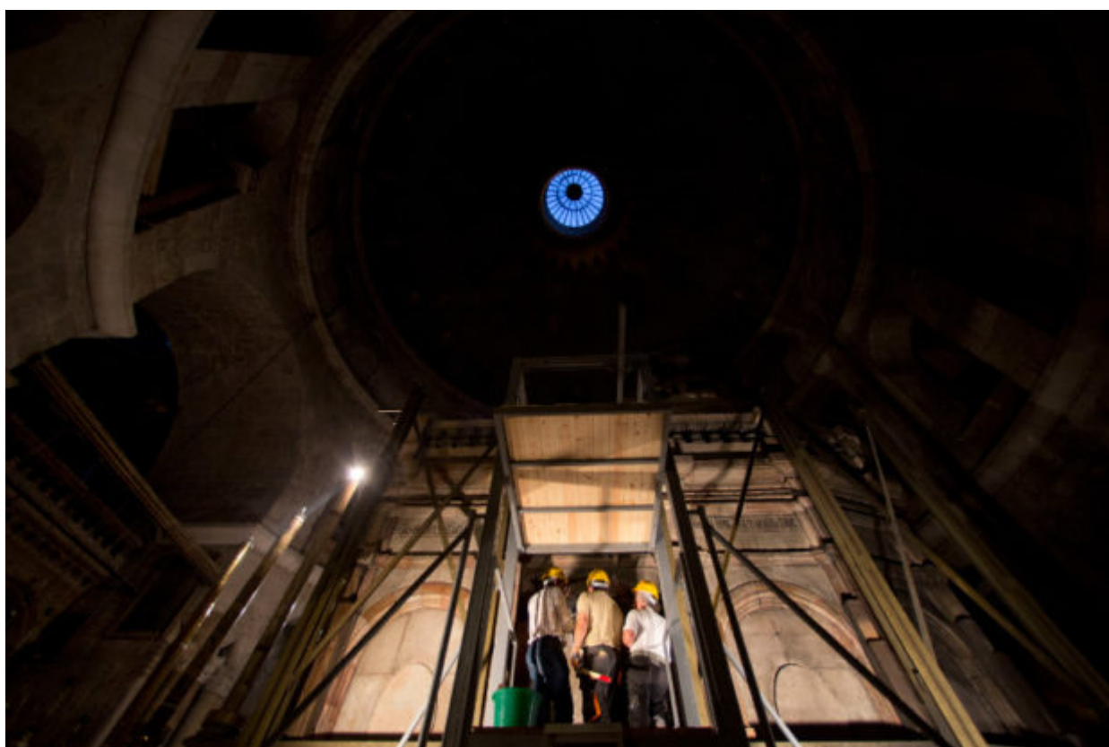
A Greek team of experts begin renovation of Jesus' tomb in the Church of the Holy Sepulchre in Jerusalem's old city, Monday, June 6, 2016. A team of experts has begun a historic renovation at the spot where Christians believe Jesus was buried, overcoming longstanding religious rivalries to carry out the first repairs at the site in over 200 years. The project, which began Monday, will focus on repairing,
